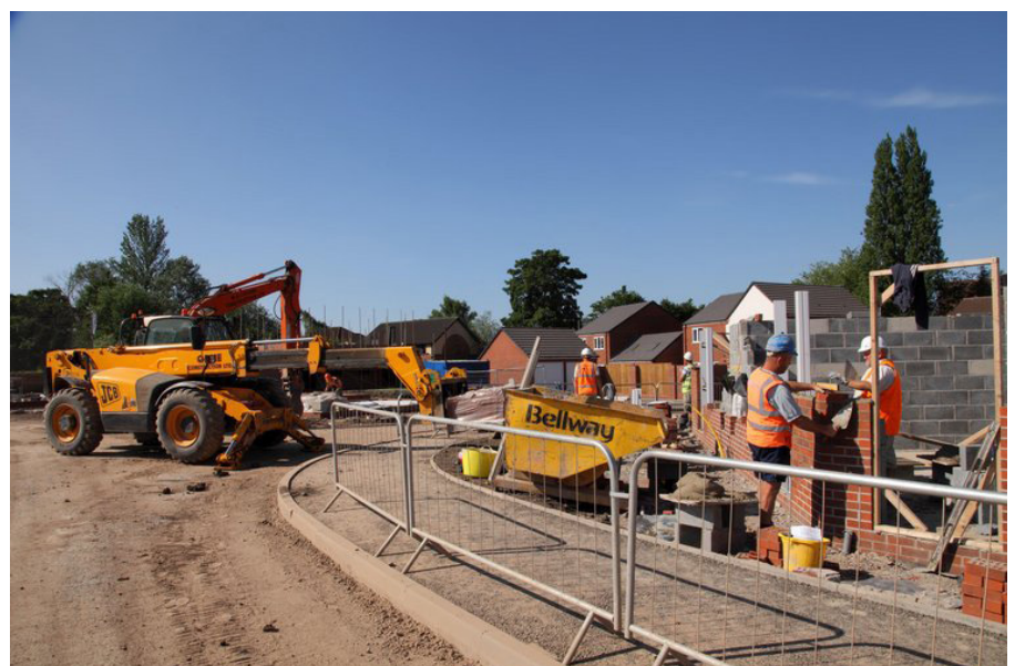
Builders and brick layers at work on a Bellway Homes construction site in the West Midlands, England, UK
